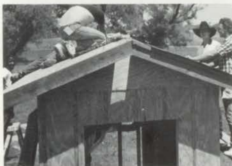
Danny Neff, Jeff Whatley, Calvin Avery, Callen Neff roofing a bathroom in Scrap Miller Park.
