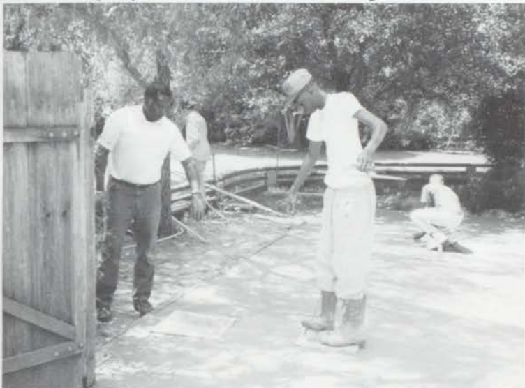
Keith Dorsey receiving instructions on how to finish concrete: Quincy Mitchell is in the background.
