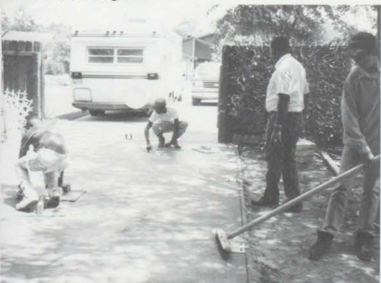
Donnie Huggins applies a broom finish to the concrete while Keith Dorsey and Quincy Mitchell are troweling the concrete.
